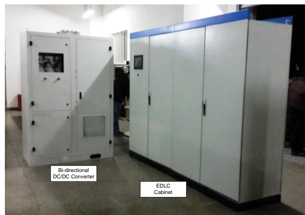
Fig.15 200kW supercapacitor energy storage system
