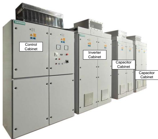
Fig.7 SES system from Siemens
